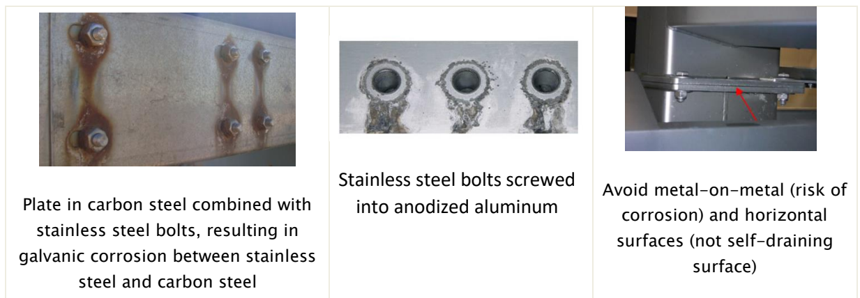
Figure 22 : examples of galvanic corrosion
